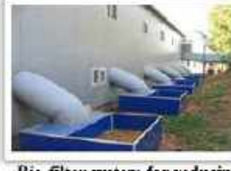
Bio-filter system for reducing malodor
