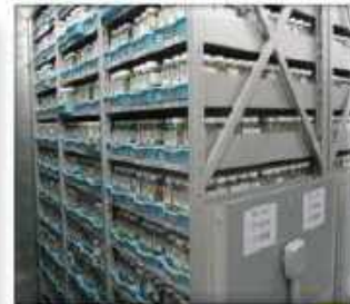
Short term storage facility
